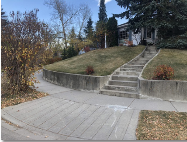
ort concrete retaining wall on corner of Salem Avenue SW and Summit Street SW.
