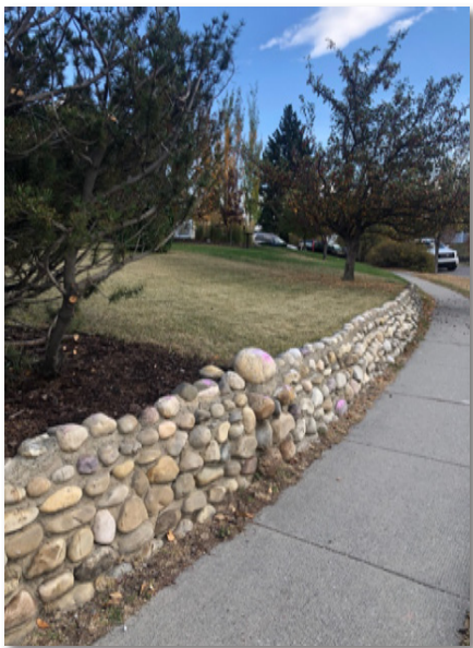
er rock retaining wall on site with grade change to the street along Summit Street SW.
